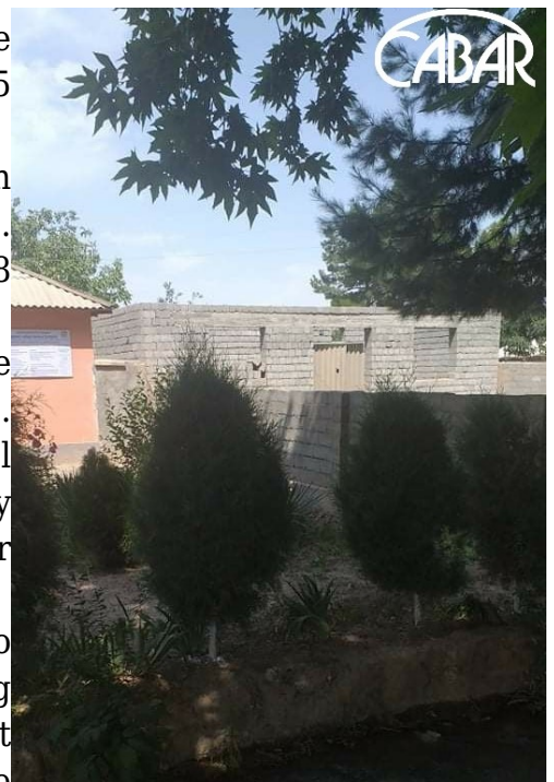
This place once was the rural club of the Marmin mahalla of the Oltinsoy district, Surxondaryo region. An entrepreneur bought it and now builds a store here. Photo: CABAR.asia
